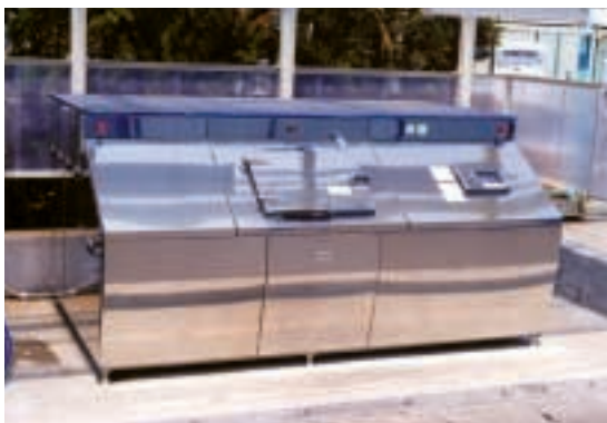
Installation of a disposal device for garbage at the Akishima Plant
