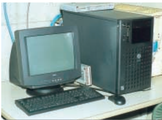
Intranet energy monitor system
