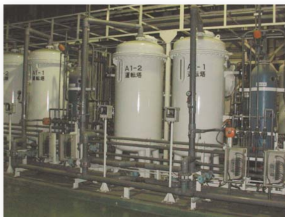
Ion exchange tank used for wastewater treatment (JAE Akishima Plant)
