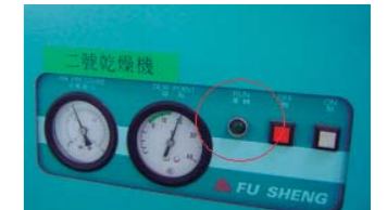
Interlock indicator on dryer
